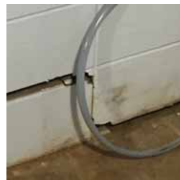
Block Wall Failure
